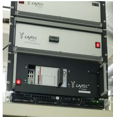
Many control units
