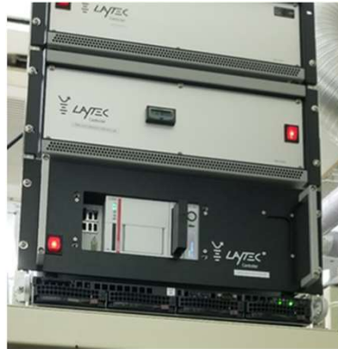
Many control units
